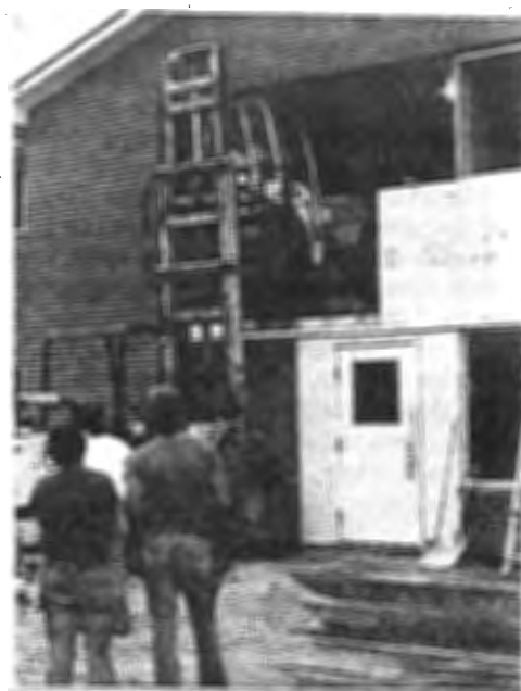
Williams Hall undergoes remodeling as a tractor is forklifted up to the second floor.
