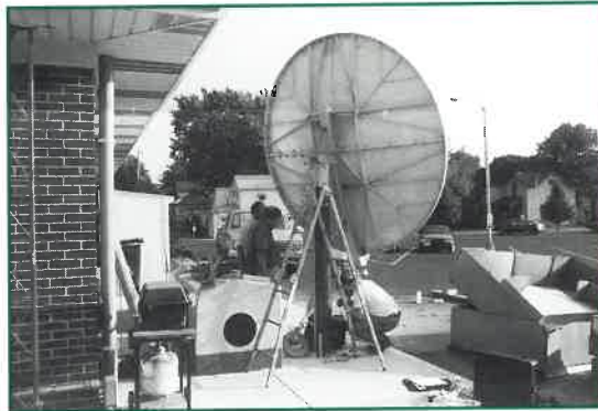
The UpLink is transmitting CDR Radio programming in CD/digital quality to all stations of the Network.
