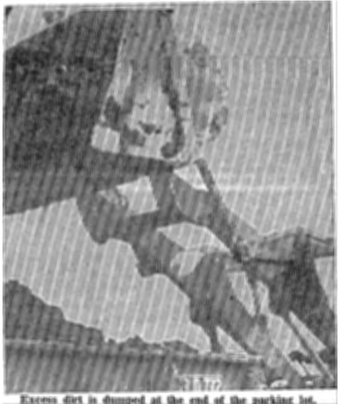
Excess dirt is dumped at the end of the parking lot.
