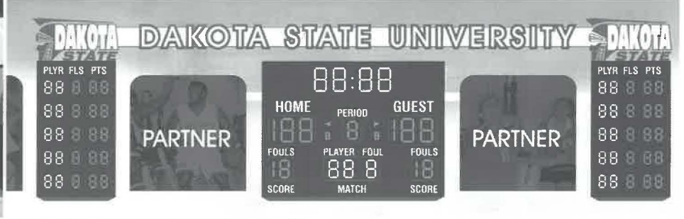
Fieldhouse - Auxiliary Endwall Scoring & Statistics Display
